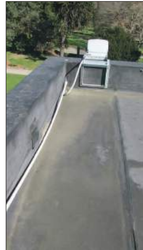
4.5 1977 Roof There are numerous ad hoc repairs made to jointing and holes in the membrane.
