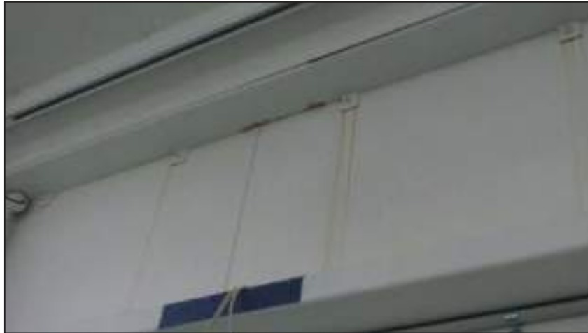
9.7 1995 Freezer panel store Persistent leaking has resulted in corrosion stains on the interior wall.
