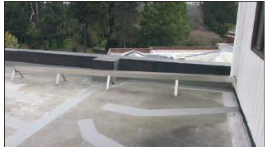
4.8 1977 Roof A temporary aqueduct built to reduce water load on this roof
