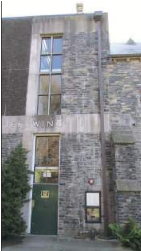
5.6 1977 Walls Part south elevation showing poorly performing area of stone wall without adequate features for water management
