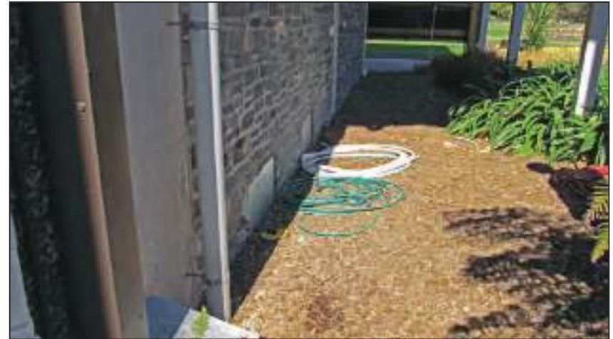
6.2 1977 Ground Ground built up above level of tanking and above penetrations in the wall
