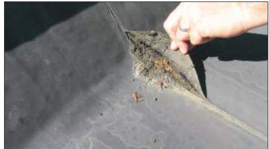
10.20 1995 General Roof Poor membrane jointing
