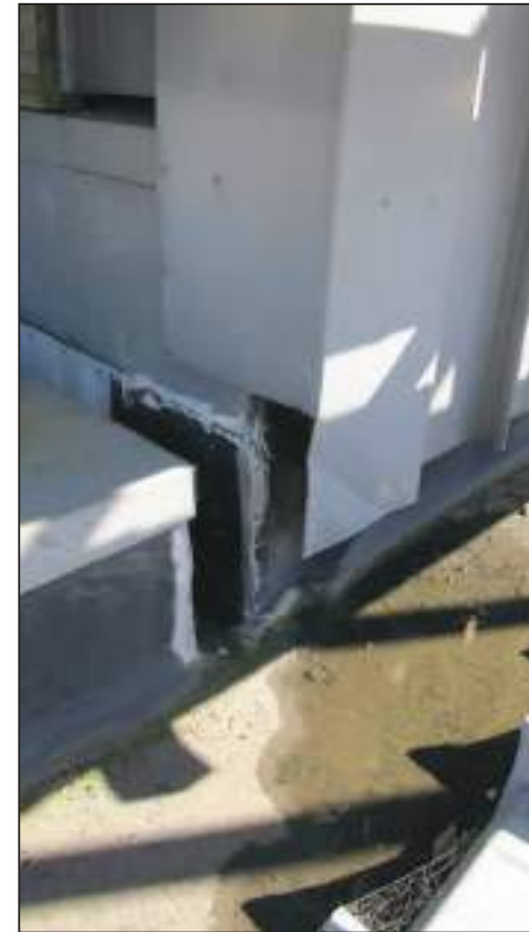
10.7 1995 General Roof Poor quality work to gutter
