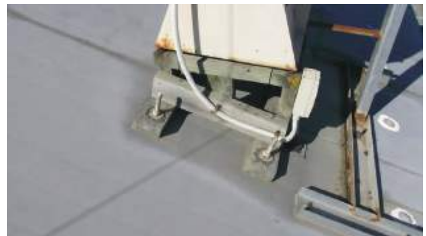
9.10 1995 Freezer panel store Very poor quality installation of services
