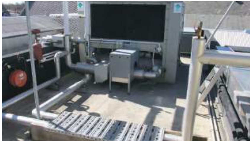
7.3 1990 The air conditioning plant platform
