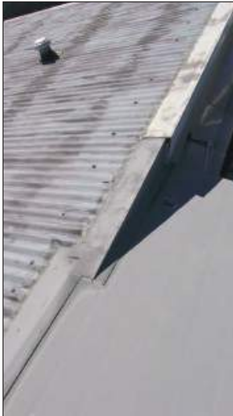
9.11 1995 Freezer panel store Poor quality flashings to adjacent roof liable to leak at any time
