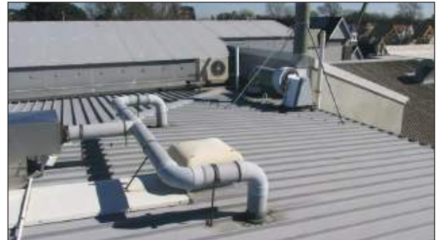
10.5 1995 General Roof Many poorly installed services in the north-western corner
