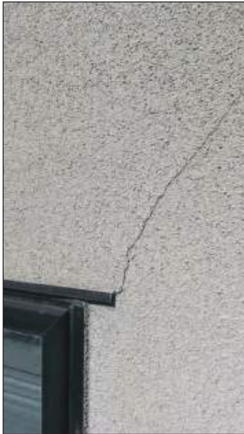
11.17 1995 General Walls Diagonal cracking from a north wall window
