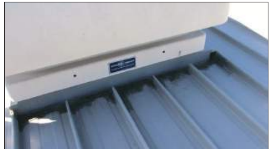
10.10 1995 General Roof There is no effective gutter above or around the ventilation penetration.
