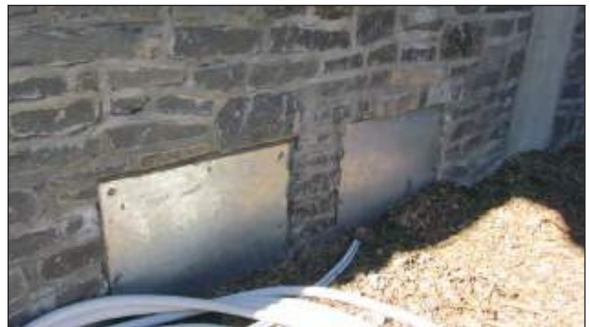
6.3 1977 Ground Ventilation or window openings have been covered over but will not be sealed adequately.
