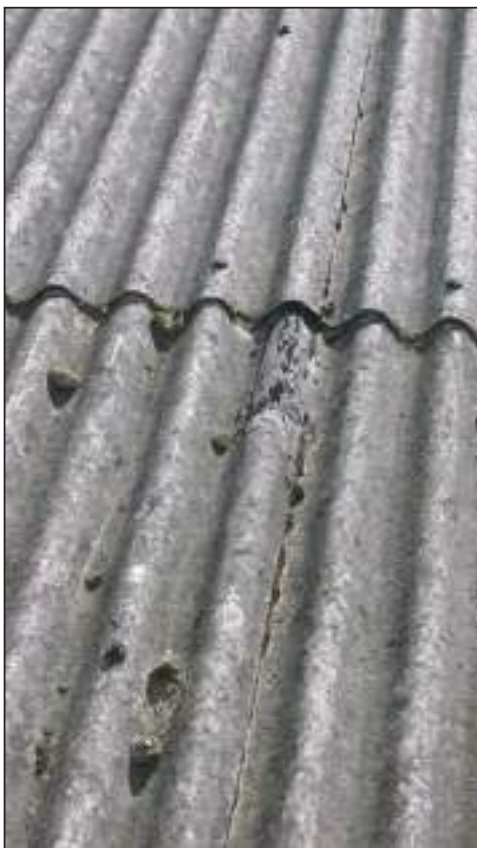
1.11 1958 Roof More examples of broken asbestos
