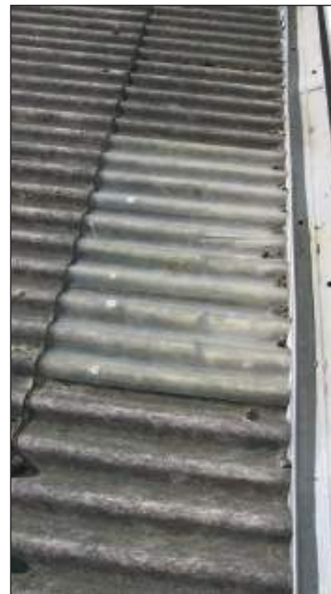
1.12 1958 Roof Areas of broken asbestos have been overlaid with acrylic sheet.
