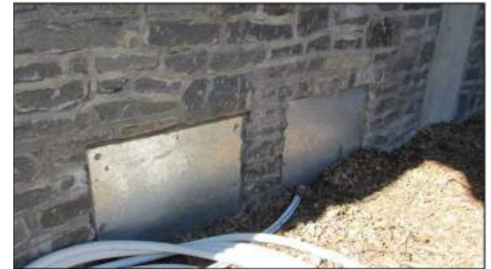
6.3 1977 Ground Ventilation or window openings have been covered over but will not be sealed adequately
