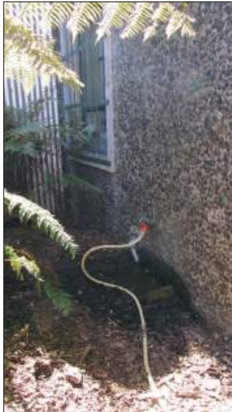
6.1 1977 Ground Ground has been built up above waterproofing and additional water load is applied to the wall.
