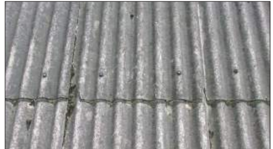
1.10 1958 Roof Examples of cracking of the now brittle asbestos
