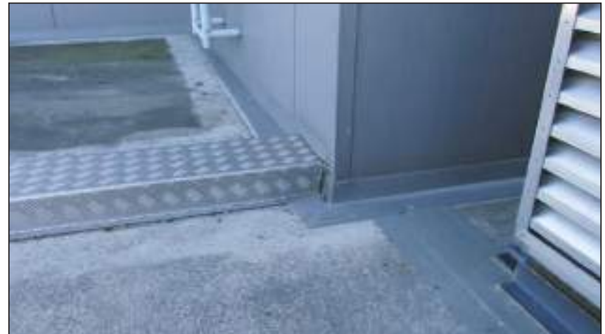
9.14 1995 Freezer panel store Complexities of connecting freezer panel building to topping slab and 1977 roof
