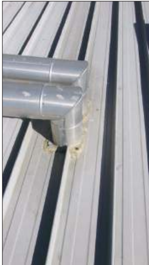
10.8 1995 General Roof Inappropriate and inadequate method of roof penetration
