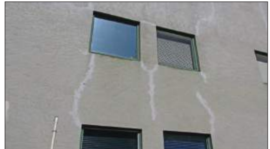
2.5 1958 Walls An example of the random cracking with temporary repair
