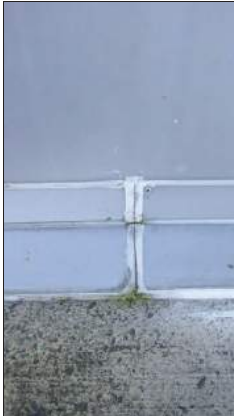
9.13 1995 Freezer panel store Flashings from topping slab to freezer panel simply butt jointed
