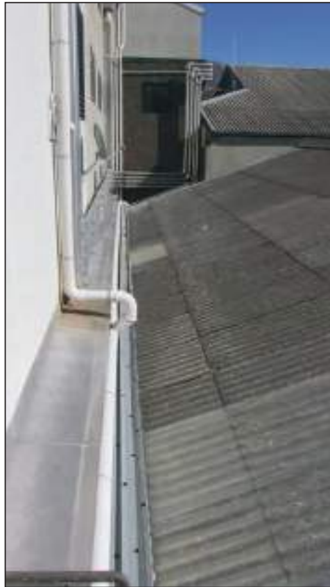
1.5 1958 Roof The internal gutters are covered over with steel with holes drilled in it.
