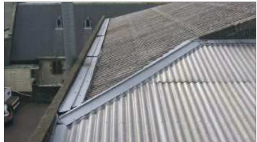
1.7 1958 Roof The western end of the asbestos roof showing the internal gutter covered over. Note that the roofing in the foreground has been overlaid with acrylic sheet.
