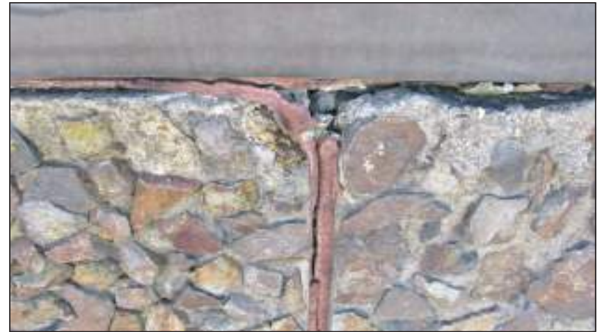
5.7 1977 Walls An example of the failed jointing between precast panels overdue for replacement
