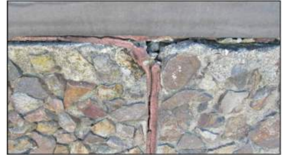
5.7 1977 Walls An example of the failed jointing between precast panels overdue for replacement
