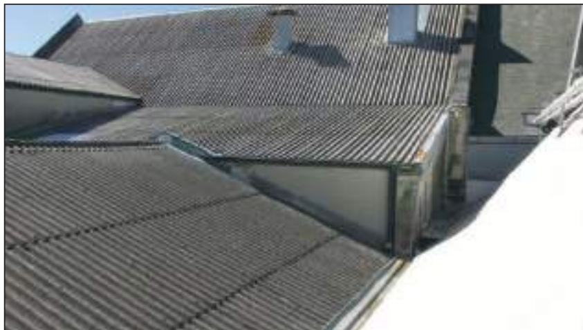
1.9 1958 Roof There are numerous complex details in this roof and the flashings will now be beyond their useful life.
