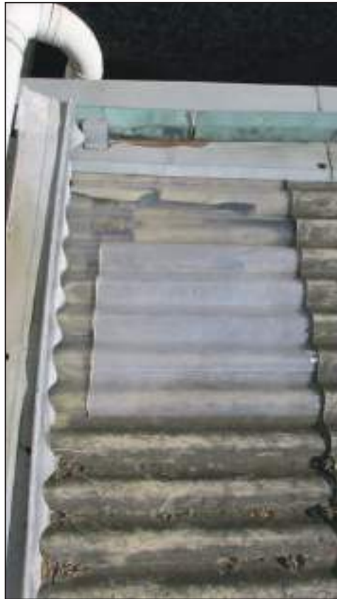
1.13 1958 Roof Areas of broken asbestos have been overlaid with acrylic sheet.
