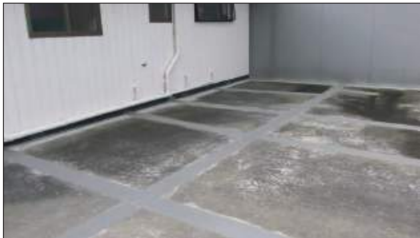
4.7 1977 Roof The connection of the topping slab to the lunchroom and freezer panel building
