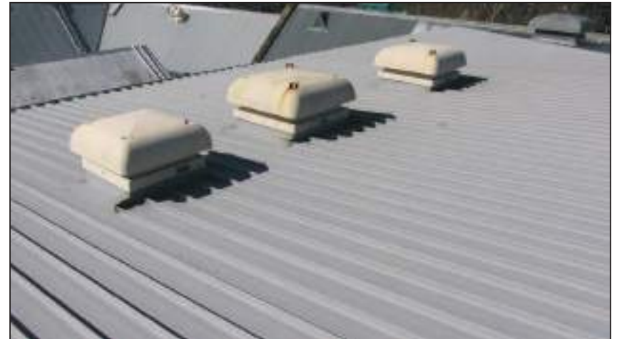
10.9 1995 General Roof Ventilation penetrations do not have appropriate water management.
