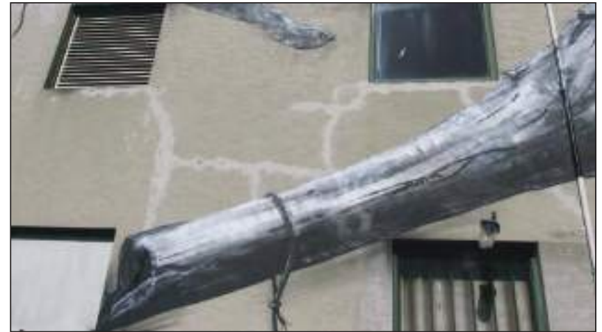
2.4 1958 Walls An example of the random cracking with temporary repair
