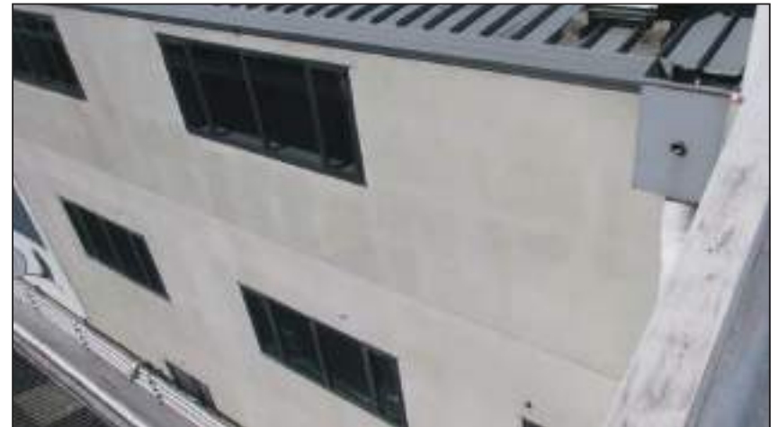
11.3 1995 General Walls North elevation fibre cement board wall in very poor condition
