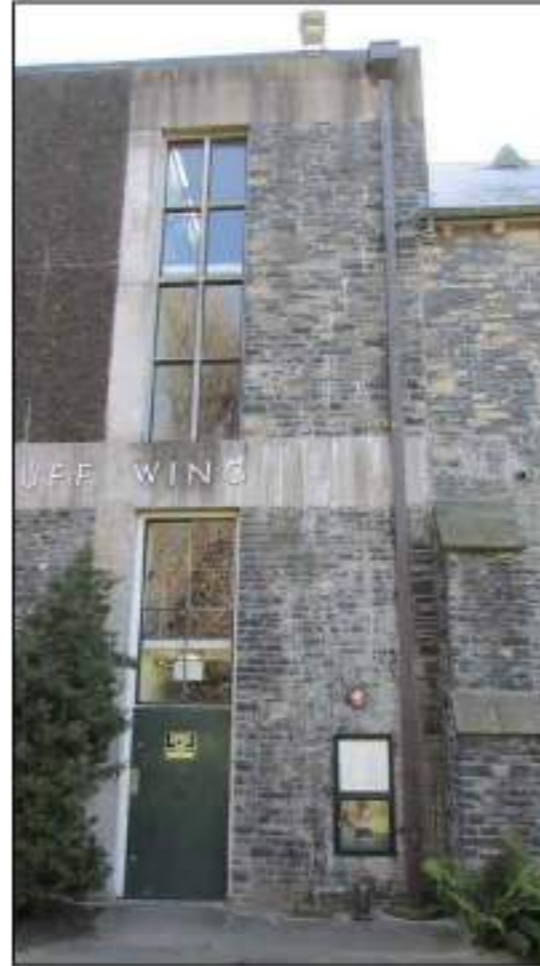
5.6 1977 Walls Part south elevation showing poorly performing area of stone wall without adequate features for water management
