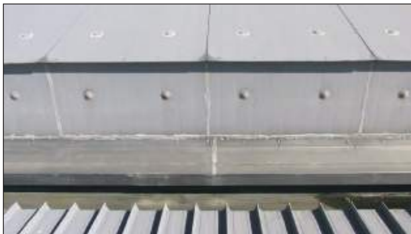
9.8 1995 Freezer panel store Poor quality connection between May 1995 and freezer panel building
