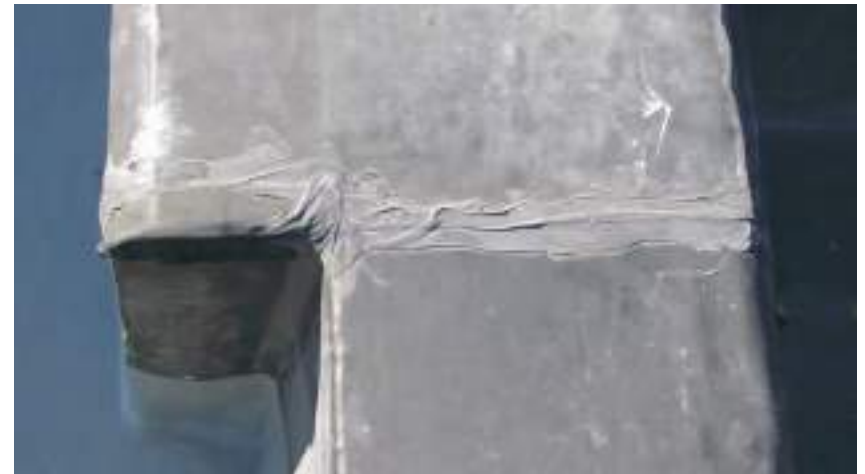
4.11 1977 Roof Incorrect jointing methods used
