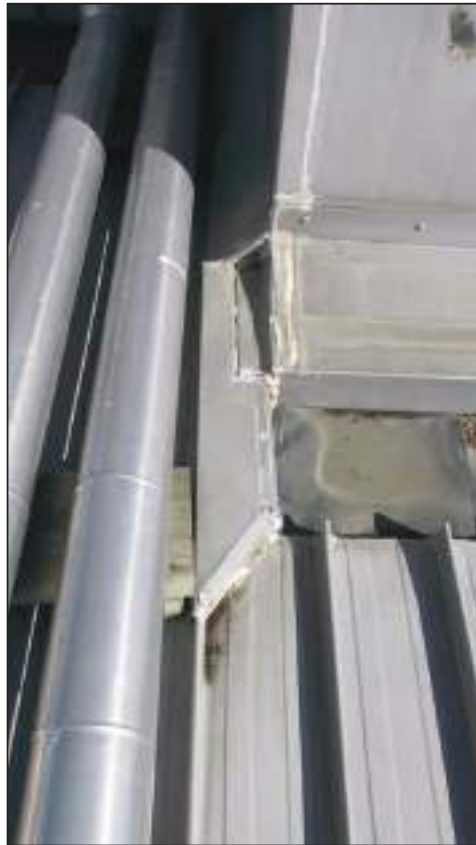
10.6 1995 General Roof Poor quality flashing and unbonded membrane and gutter
