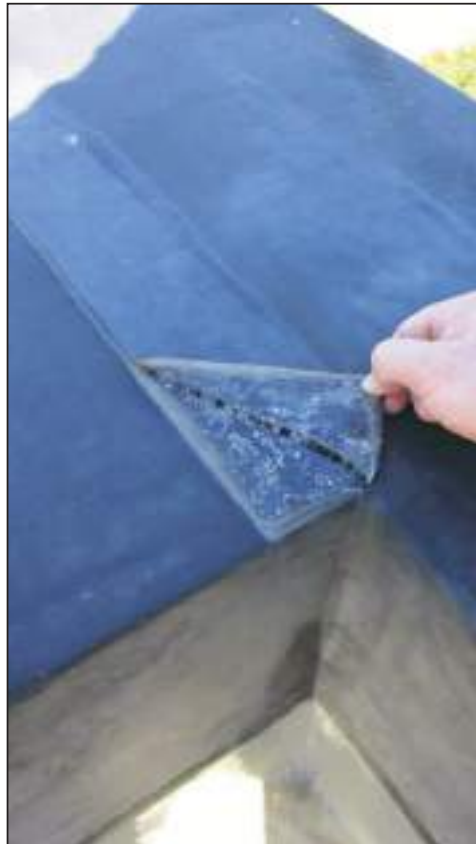
4.10 1977 Roof Incorrect jointing methods used
