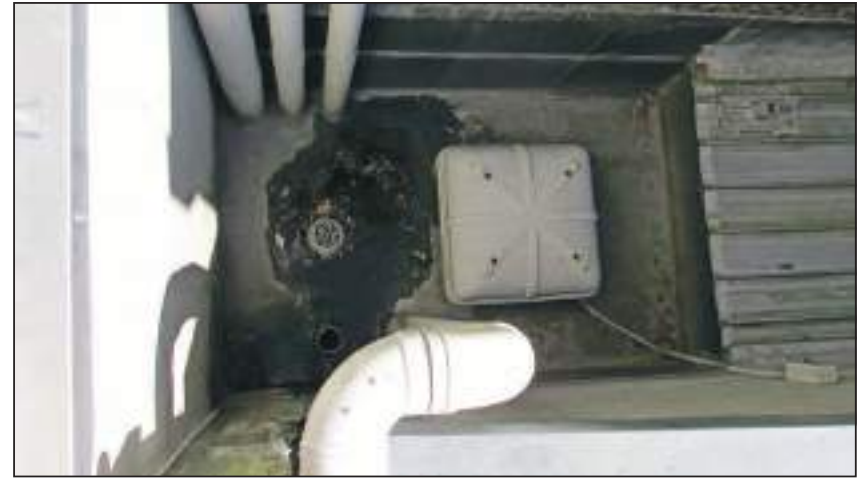
1.16 1958 Roof A closer view of the sump that poses a particular hazard to the Museum
