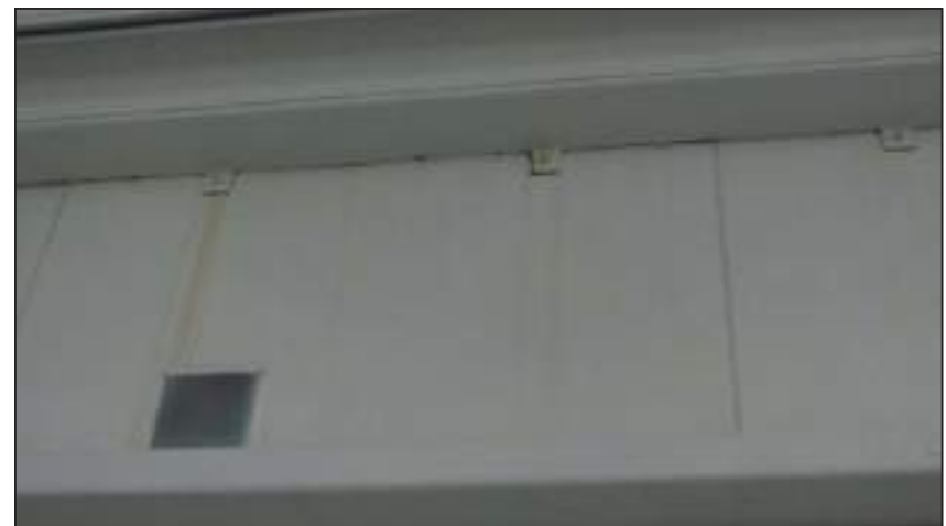
9.6 1995 Freezer panel store Persistent leaking has resulted in corrosion stains on the interior wall.
