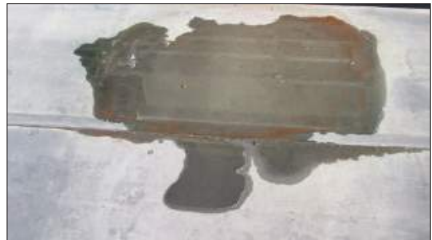
10.21 1995 General Roof Fixings of plywood are applying upward pressure to underside of membrane.
