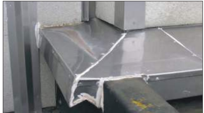
11.18 1995 General Walls Flashings made from good quality and durable material but installed so poorly that they are ineffective
