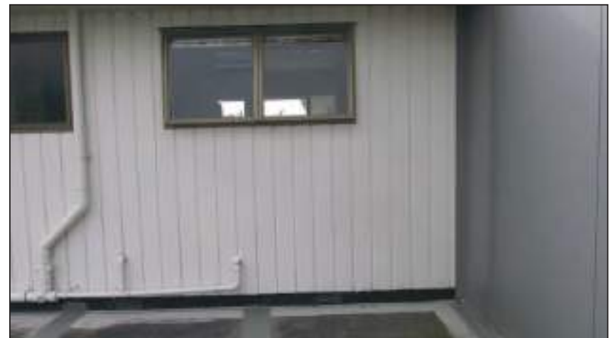
8.6 1995 Staffroom South elevation showing decayed weatherboards
