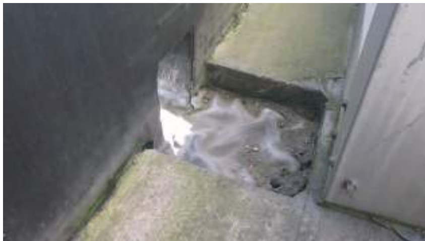
7.4 1990 Deteriorated butyl rubber at the drainage outlet to this area
