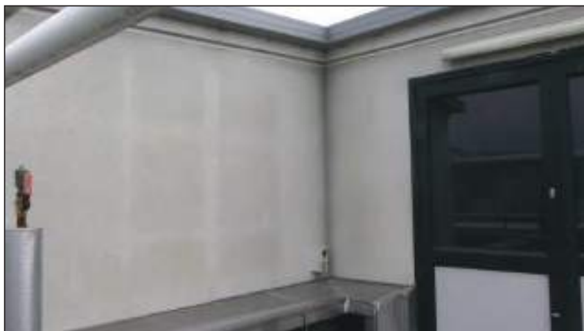
11.8 1995 General Walls Eastern corner of building. Note how the location of the timber framing can be seen due to the staining patterns on the texture-coated fibre cement board.
