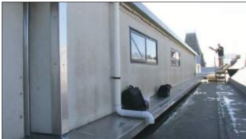
11.2 1995 General Walls Wall framing visible through the texture coated fibre cement wall cladding
