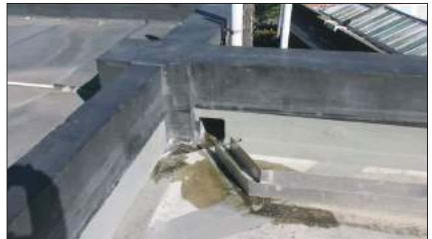
4.9 1977 Roof A temporary aqueduct built to reduce water load on this roof
