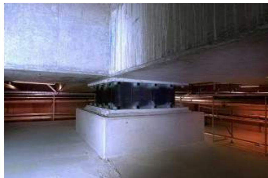
Christchurch Women's Hospital base isolator between foundation slab and basement (Image: Holmes).
