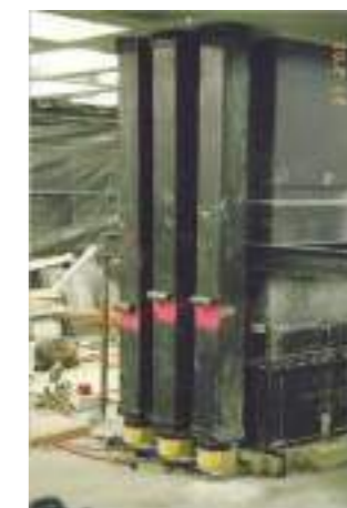
Level 0 props and jacks used while cutting the columns (image: 2004 NZSEE conference)
