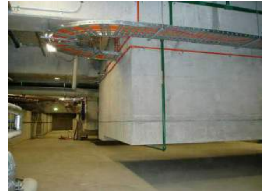
Christchurch Women's Hospital lift pits suspended into the basement from the superstructure.
