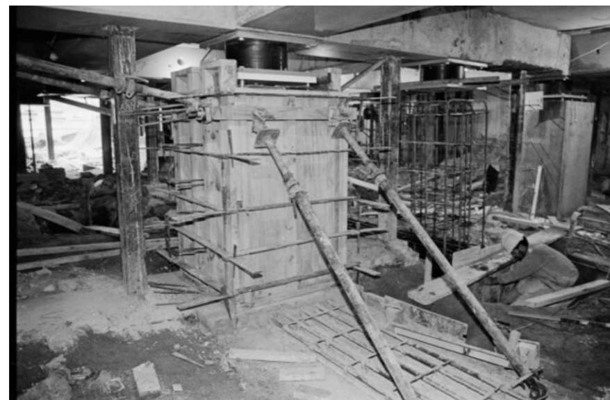
New Zealand Parliament building base isolators being retrofitted. Section swer cut from the existing foundation columns. (image: 1993 Dominion Post)
