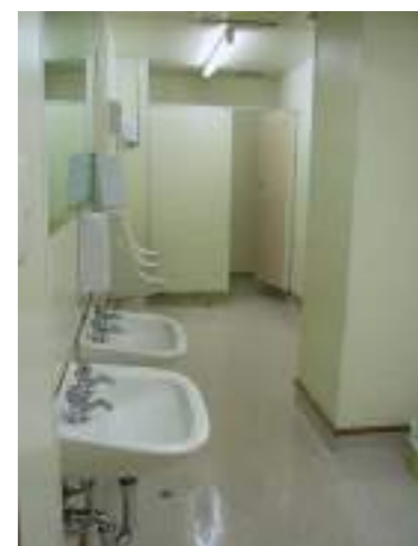
Current public toilets - not enough stalls and in poor conditions that needs urgent upgrade
