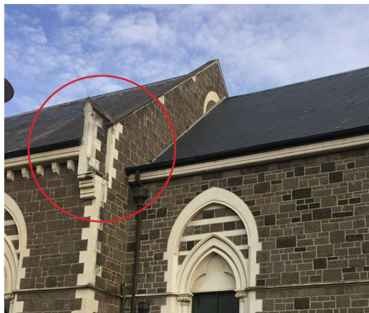
Image 23: Eastern corbel detail of the 1877 Wing. The redevelopment will unveil the western corbel to public view. If a physical connection were to be required, due to the detailed nature of the corbel it is
