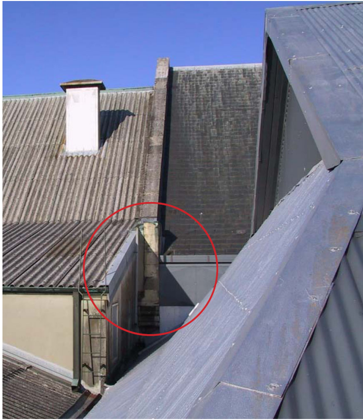
Image 22: Existing 1877, 1882, 1958 roof junction. This highlights the complexity of flashing (both for seismic and waterproofing) where multiple buildings come together. This indicates the physical impact to heritage fabric and legibility of heritage form (source Athfield Architects Ltd, 2000).
