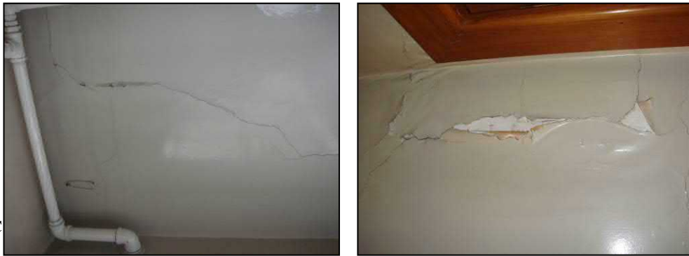
Crack and paint lifting in the wall of the upstairs servery.
