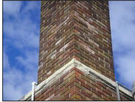
Efflorescence in chimney. Note also erosion of limestone string course (DPAL).
