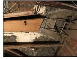
(5) View to the 1872 east wall with trachyte stone work, as seen from the 1877 building roof space.
