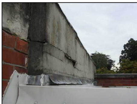
Damage to parapet with erosion evident (DPAL) membrane (DPAL)
