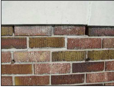
Crack in stringcourse with evidence of loss of mortar in brickwork. (DPAL)
