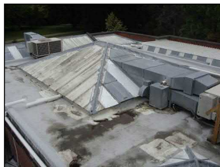
Evidence of water pooling and patched surface
