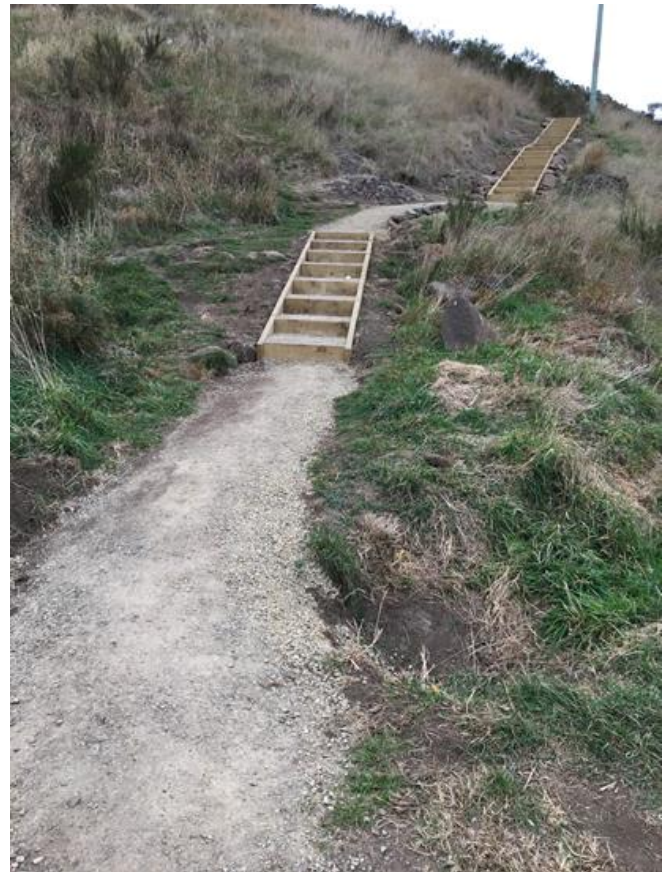
Two flights of wooden stairs and material including shingle brought in to form urbanised path
