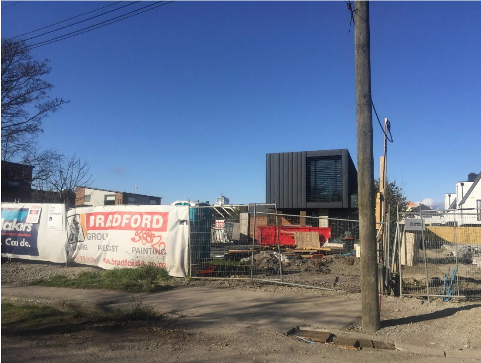
View south from Gracefield Avenue towards the site. The dwellings at 3/363 and 6/362 Durham Street North within close proximity of the site can be seen to the right.
