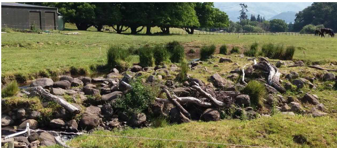
Figure 13 Storm debris deposited by Robinsons Bay stream immediately below Sawmill Road bridge
