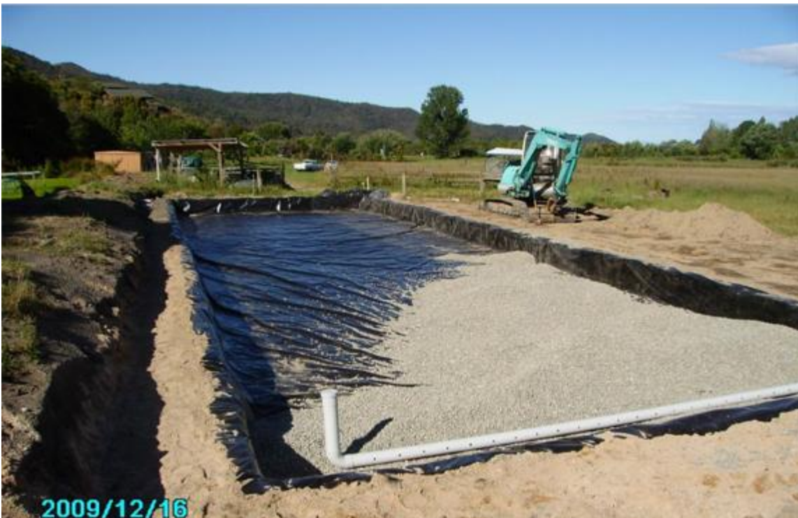
Figure 5-4 Construction of a Subsurface Flow Wetland (at Abel Tasman courtesy of Cameron Gibson and Wells Ltd)
