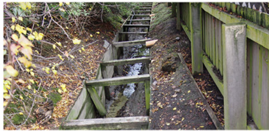
2 Existing Lydia boxed drain
