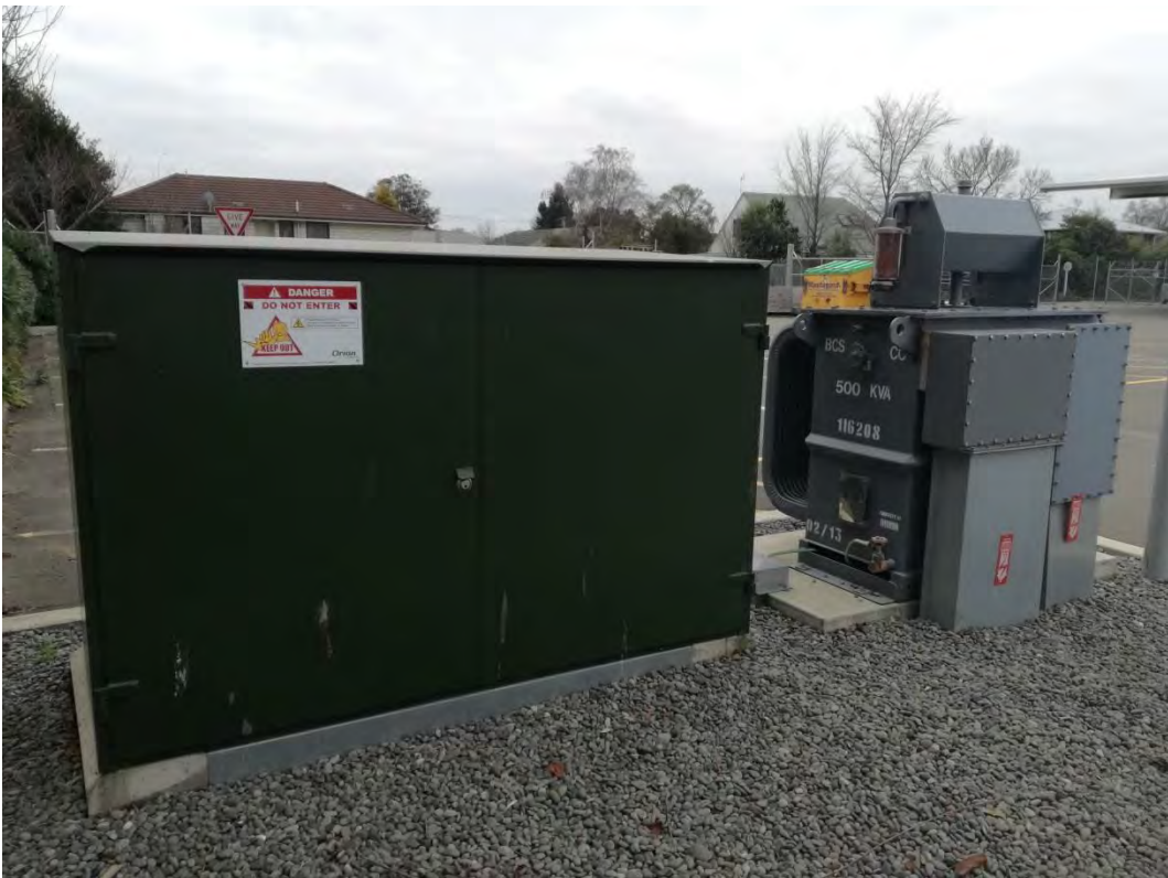
Photograph 10: Transformer located in the west of the site (west of 171 Main North Road at 165 Main North Road).
