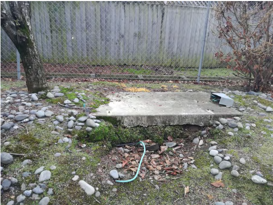
Photograph 8: View of concrete slab between the drain and the access road in the west of the site.
