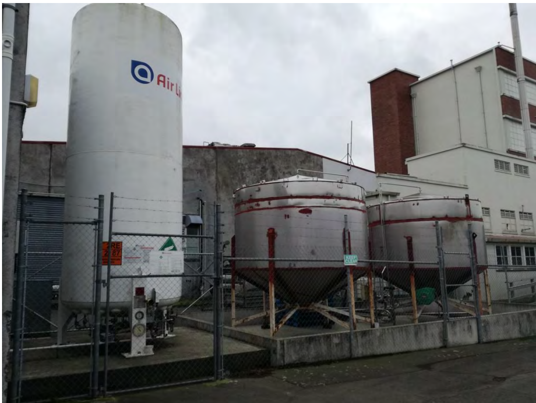
Photograph 12: Tank containing liquid carbon dioxide adjacent to two unlabelled tanks (171 Main North Road).
