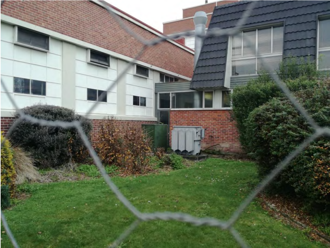
Photograph 5: Transformer located in the east of the site (171 Main North Road).
