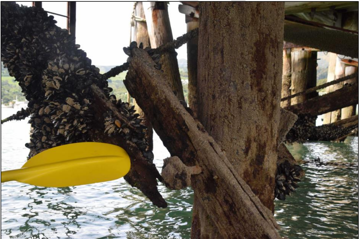
Photo 33 Broken timber brace.
