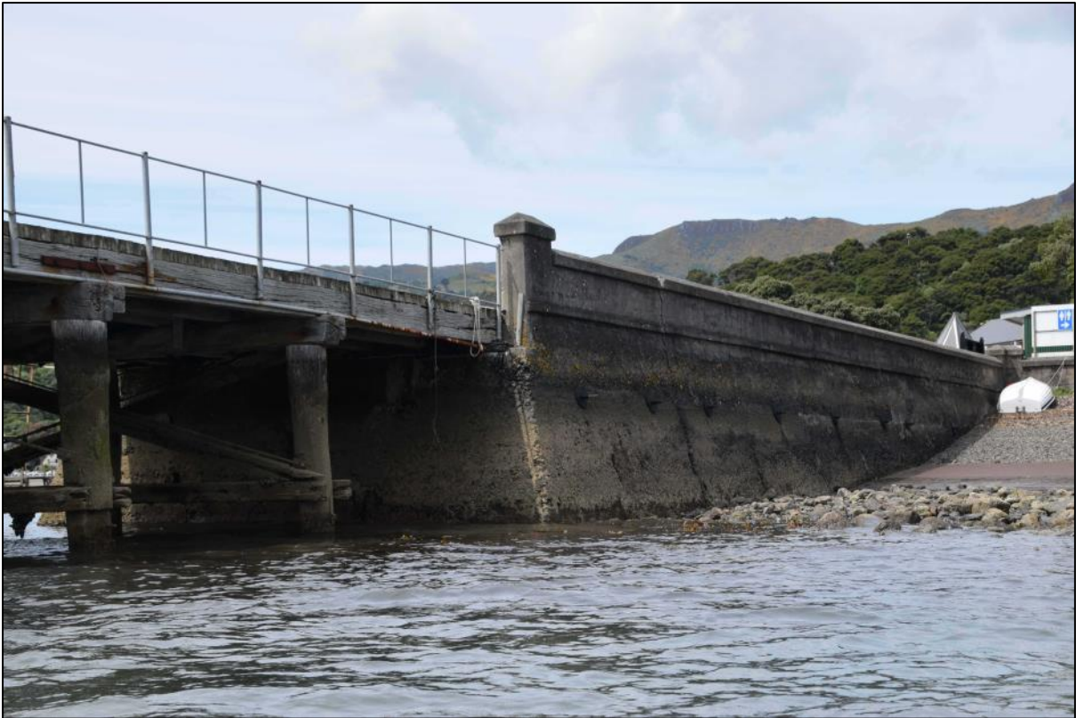
Photo 24 The junction of the abutment, and its concrete wall, and the start of the timber wharf structure on the south side. Galvanised steel railings have replaced the painted timber railings since 1973.
