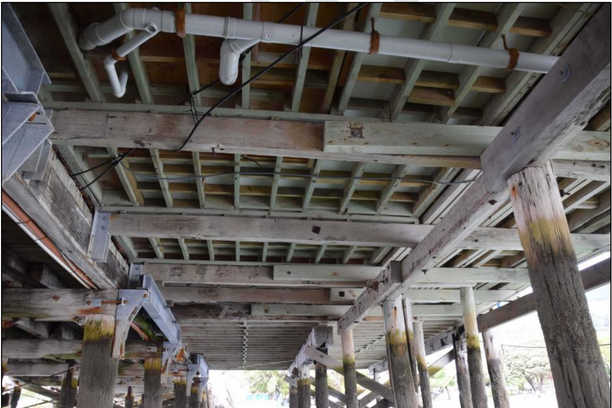
Photo 43 As Photo 42 (looking east), but showing in more detail two different periods of modern floor framing (foreground and distance).
