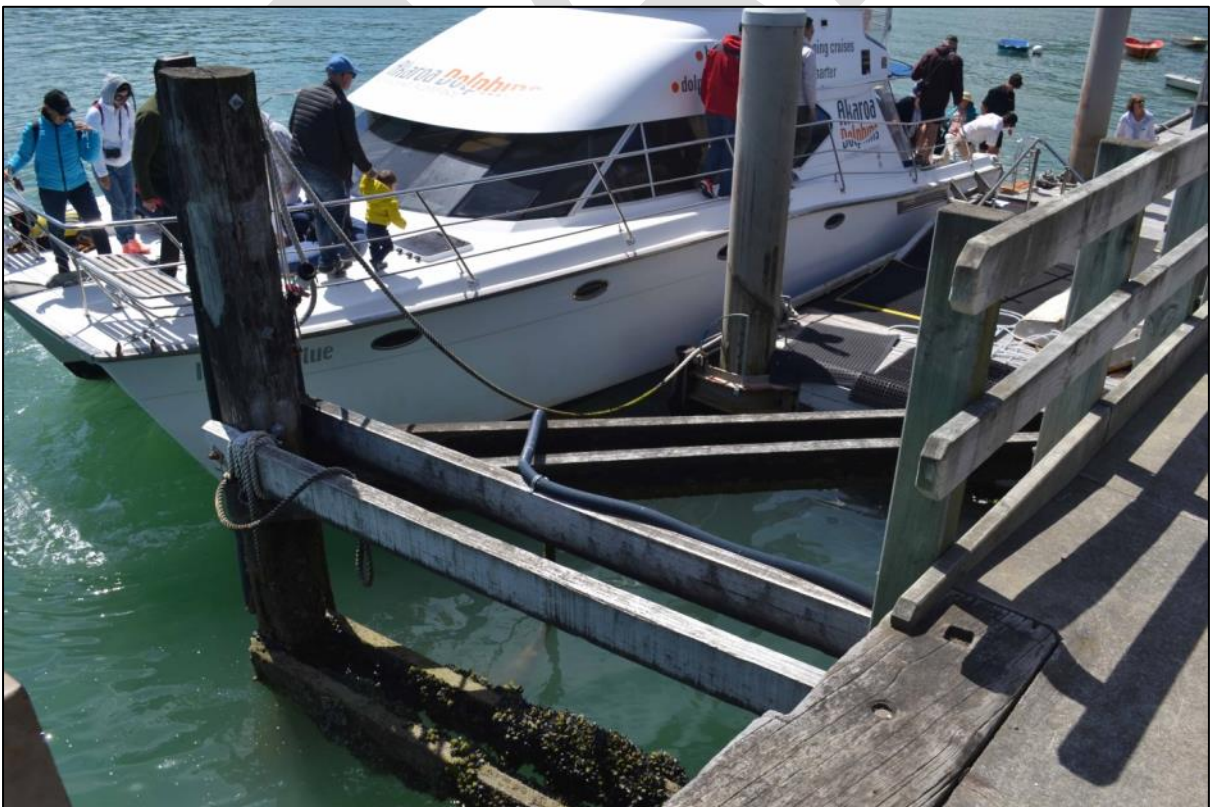
Photo 9 This older pile on the left appears to relate to the former projecting platform and main steps to water level that previously existed on the north side of the wharf.
