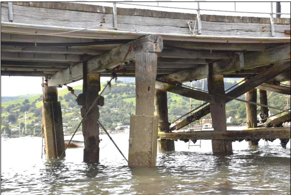
Photo 25 The same bent as in Photo 6, but from the south side. Both outer piles have 'jacket' repairs and the bent is missing its original horizontal brace. The diagonal timber braces have been cut off and replaced by steel rods.
