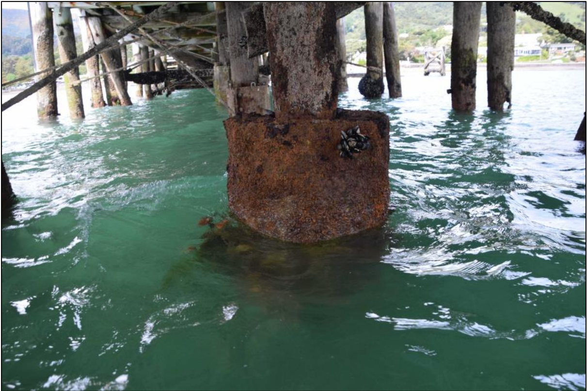
Photo 26 A 'jacket' repair to a central pile under the western end of the wharf. The pile has continued to erode above the jacket.
