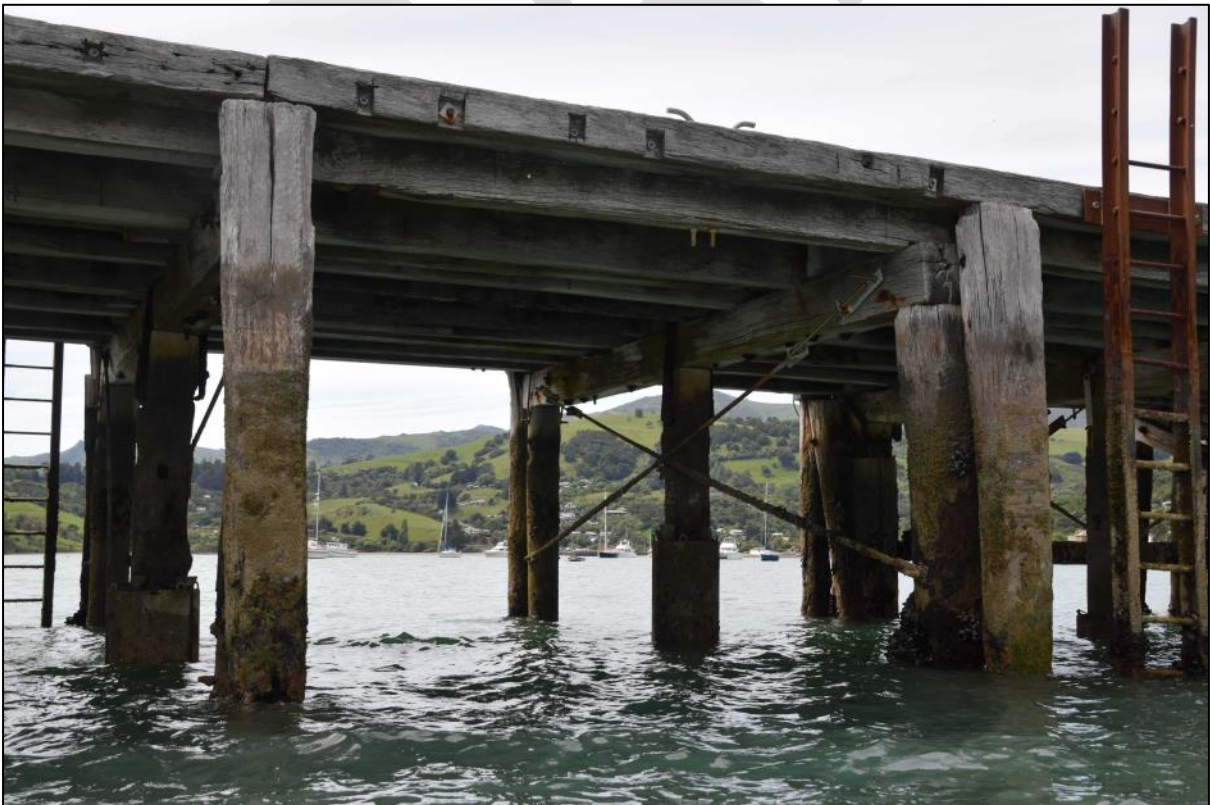
Photo 13 Here the original timber cross-braces to the bents have been replaced with modern steel bracing rods and a number of the piles have had repair 'jackets' encased around their lower sections.
