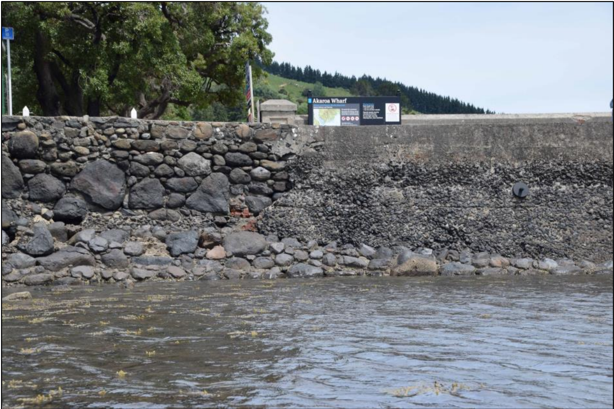
Photo 2 The north face of the seawall at the junction of the abutment and Reserve.
