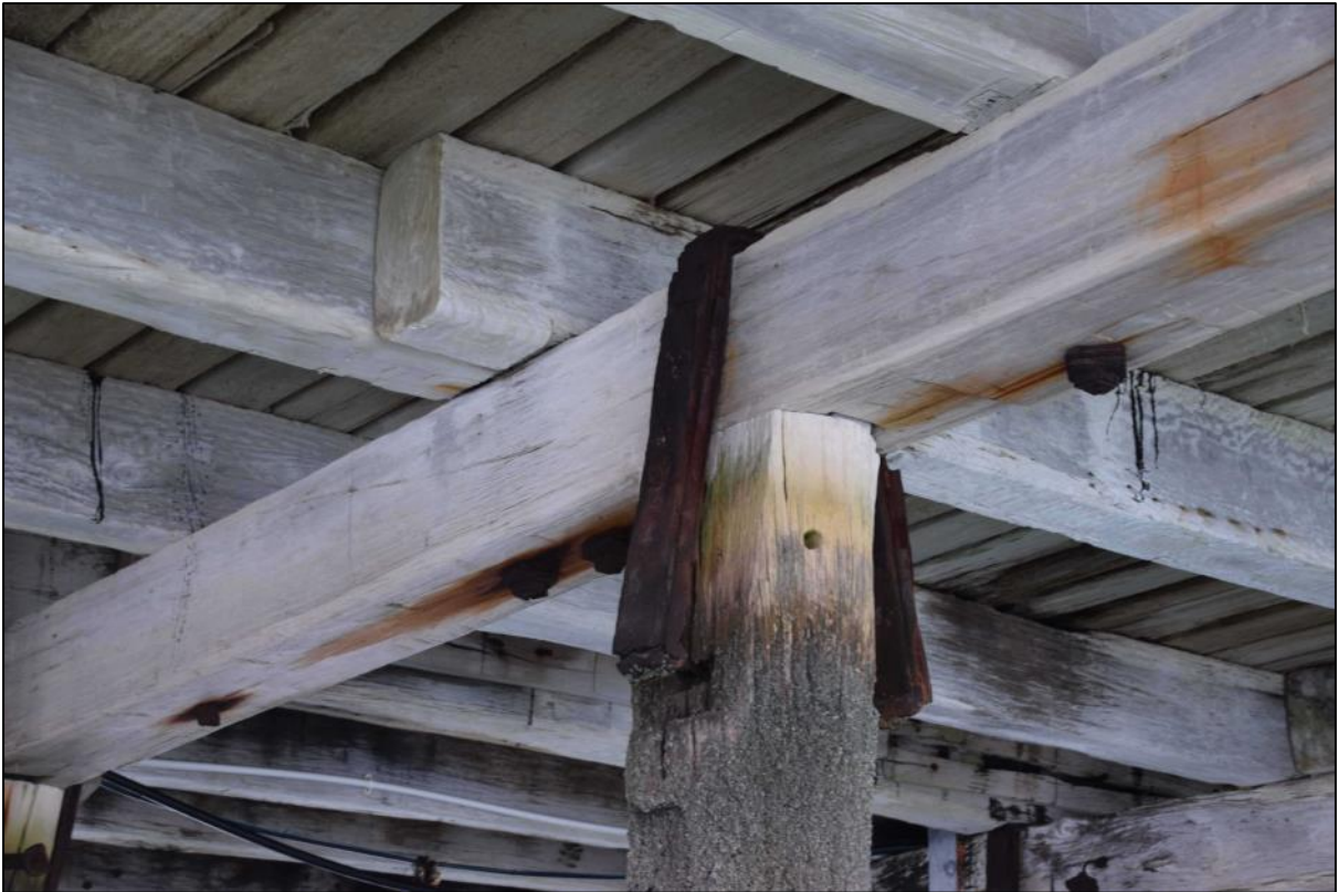
Photo 18 Close-up of the pile head on the right of Photo 17 showing the original wrought iron strap connection with the pile cap beam – now corroding/delaminating and separated from the pile head.
