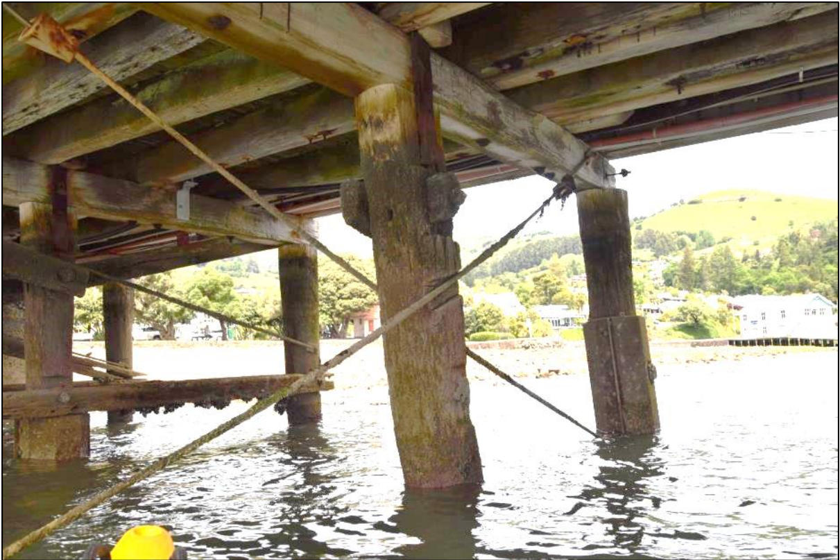
Photo 6 An example of repairs and alterations to a bent – original timber bracing cut off either side of the central pile; diagonal steel braces installed; and a steel jacket added to the right-hand pile.
