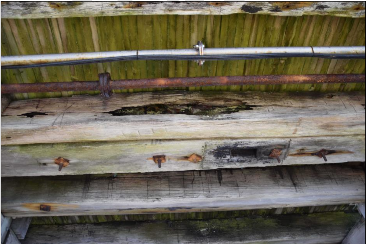
Photo 5 Clear evidence of decay in a timber stringer at the eastern end of the wharf.
