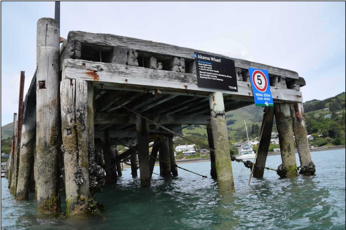
Photo 12 The outer/west end of the wharf clearly showing the original construction, although with some replacement tanalised piles. Along the top of the piles is the timber pile cap (beam). On top of that are the stringers and running parallel to the cap is the timber kerb with the timber decking behind it. On the far left and far right are fender piles and each corner has an inner bracing pile.
