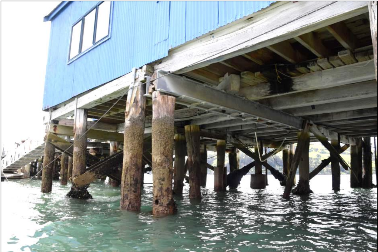
Photo 20 Steel beams either side of a pile cap. It is possible that the short section of diagonally-laid timber beam (cut face towards the camera) on top of the steel strengthening is where the original wharf structure narrowed at the end of the former wharf sheds.
