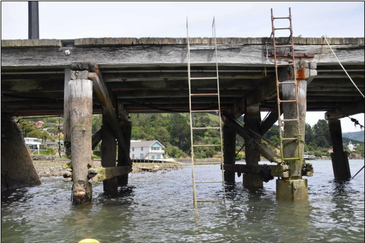
Photo 4 Three pile 'bents' under the eastern end of the wharf close to the abutment. Note the diagonal, timber braces, horizontal timber ties beneath the braces, and later steel rod braces. The original construction can be clearly seen here with timber pile caps (beams) running along the heads of the three piles in each bent and the timber stringers and decking on top. There are no fender piles to this part of the wharf. Ladders are a late 20th century addition.
