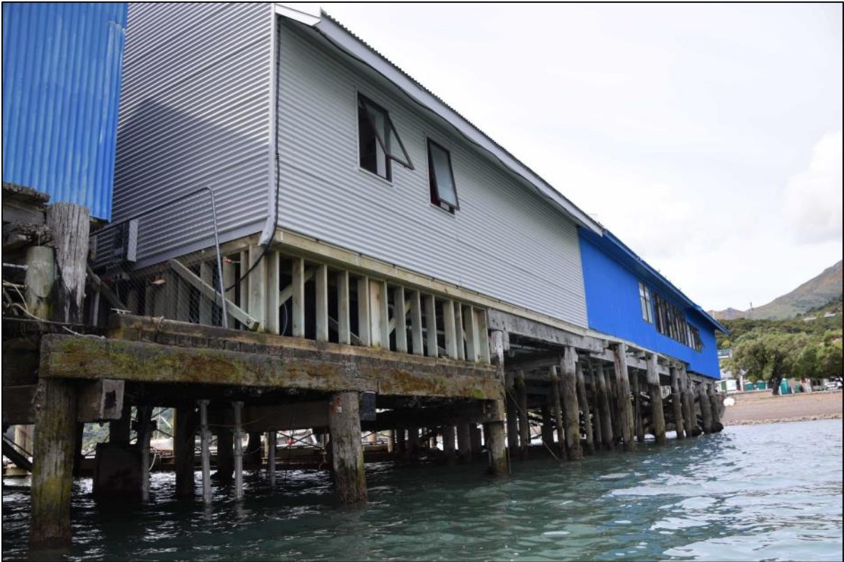
Photo 22 showing the lowered deck area (Photo 21) accessed by timber steps between the two sheds. Note the steel props under the lowered deck.
