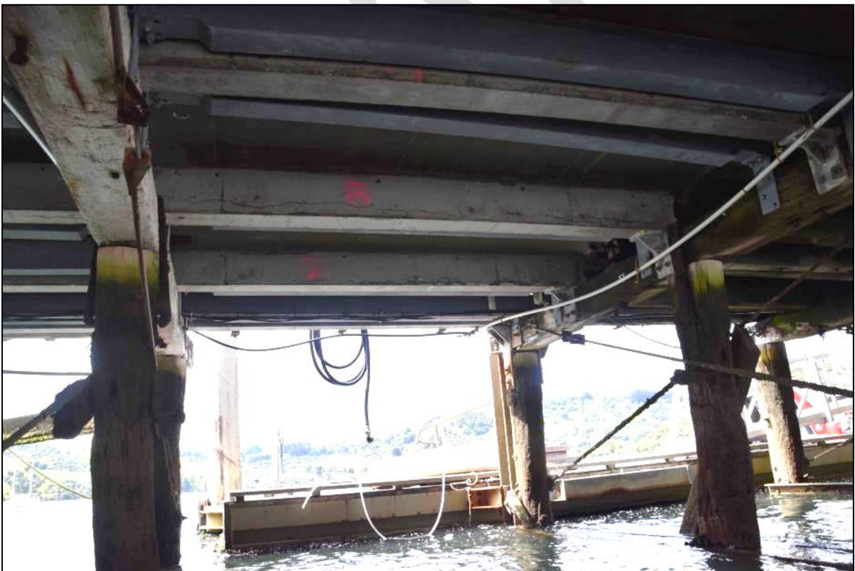
Photo 41 A close-up of inserted concrete and steel beams (Photo 40) – some of the concrete beam are cracked. Poorly restrained and concealed modern conduits.
