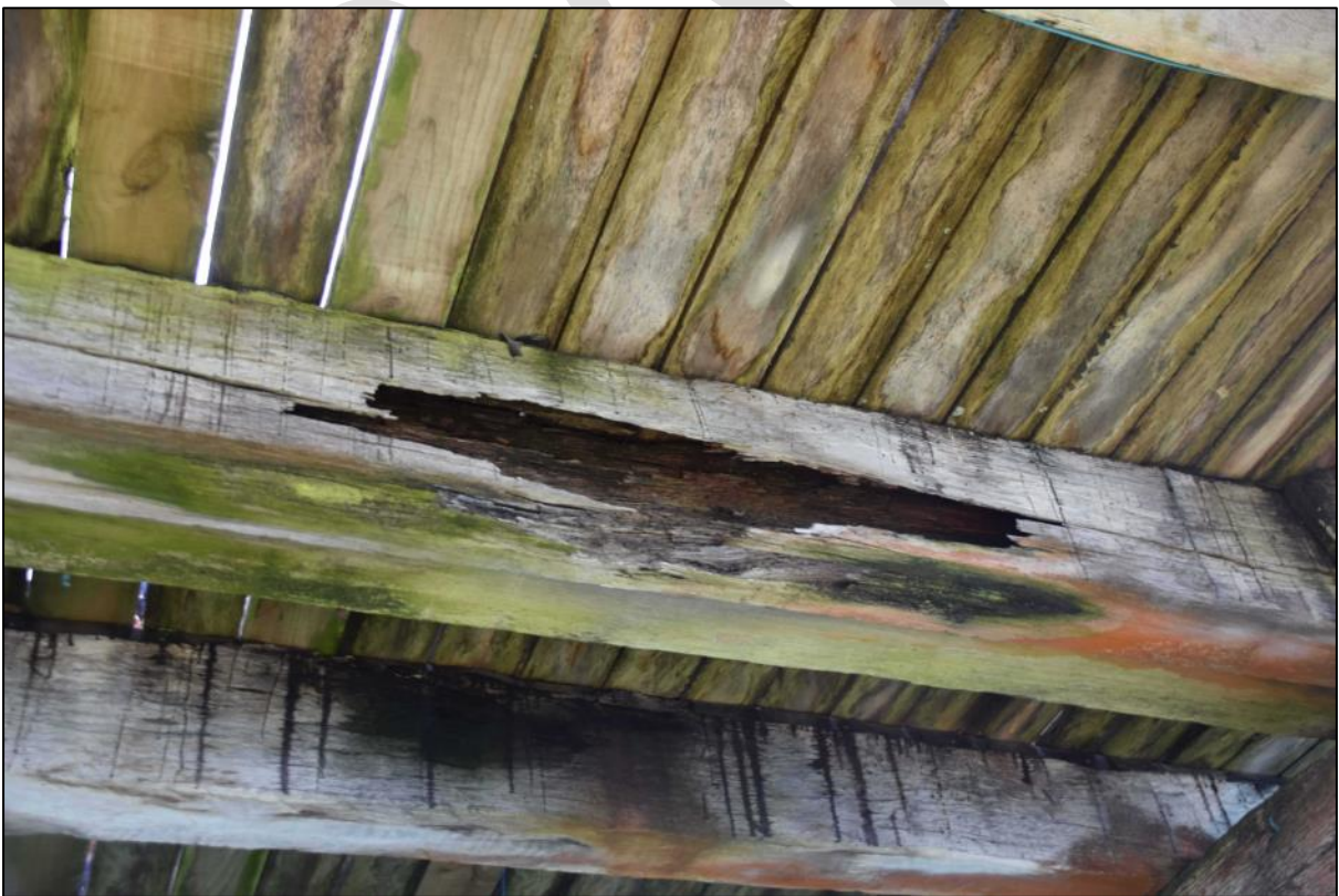
Photo 31 A large area of decay in one of the stringers close to the modern steps toward the western end of the wharf.
