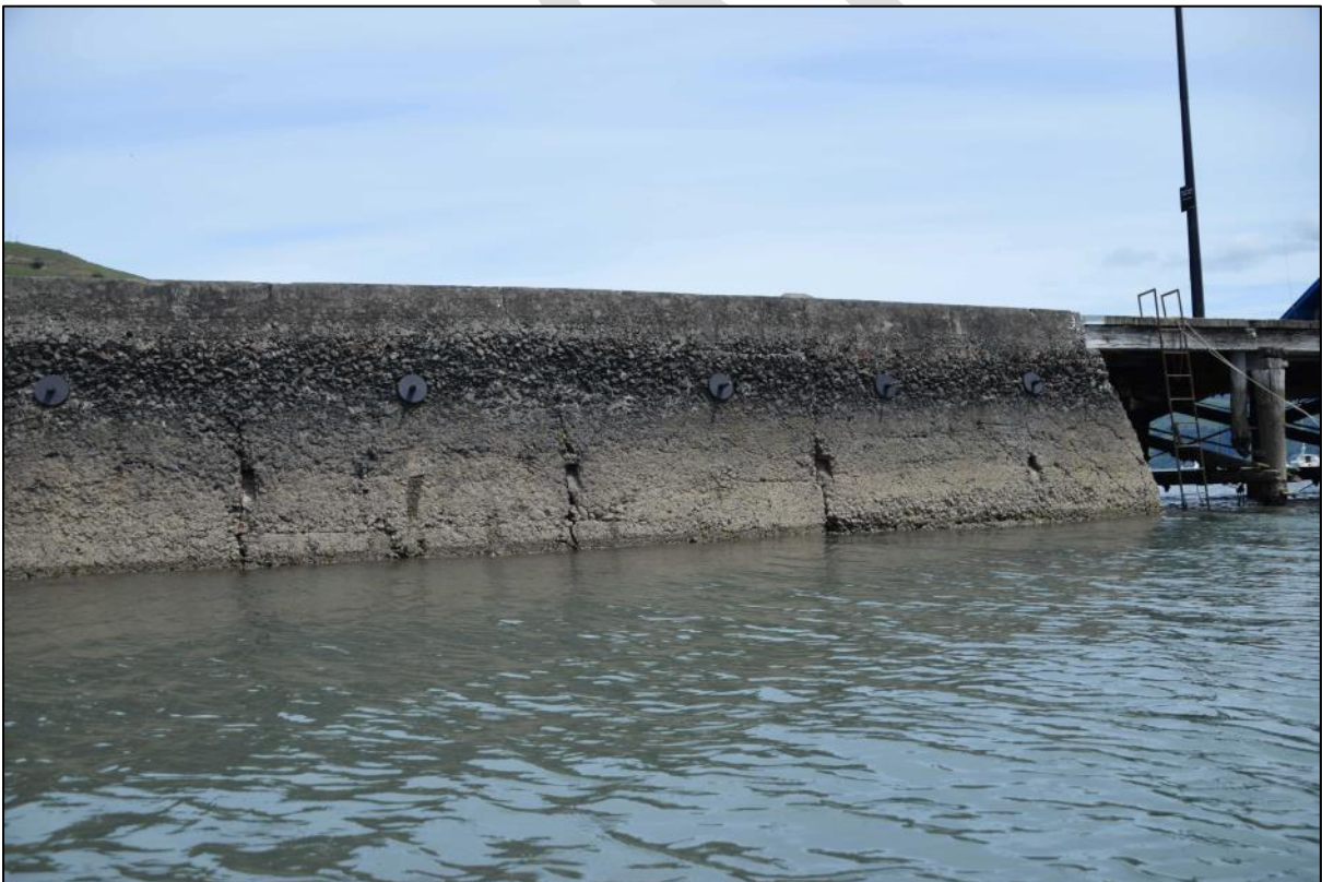
Photo 3 The outer north wall of the abutment with drainage holes, circular pattress plates to the end of the tie rods and many cracks in the masonry.
