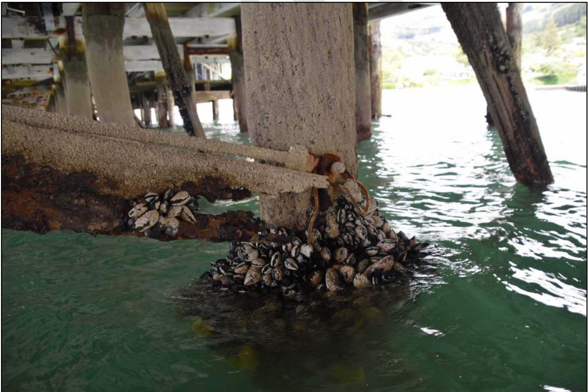
Photo 35 Broken/corroded steel brace.
