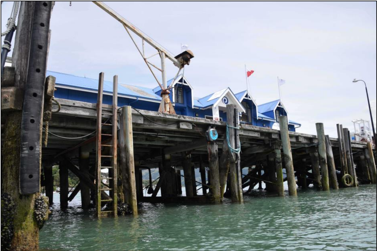
Photo 8 The north side of the wharf beyond the floating pontoon with modern ladders and replacement tanalised fender piles. The width of the wharf has substantially widened to accommodate the late 20th century sheds. Refer to Photo 9 below regarding the pile in the foreground on the left of the image.
