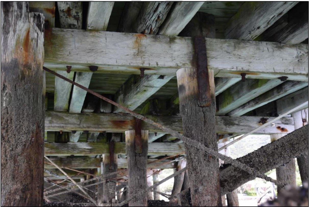
Photo 29 original wrought iron strap connections between the central piles and their pile cap. The joints also have a mortice and tenon.
