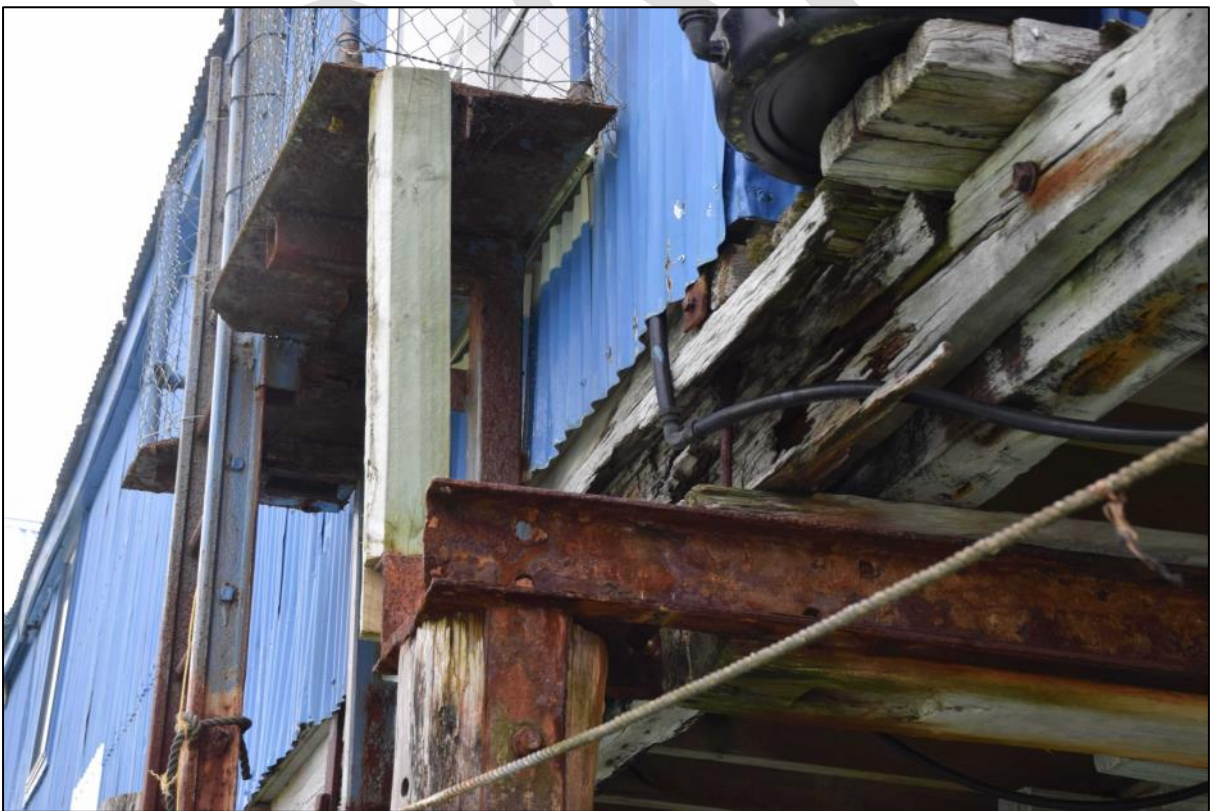
Photo 19 Timber decay and corrosion at the junction of two of the modern sheds (south side approx. 16th bent from the abutment).
