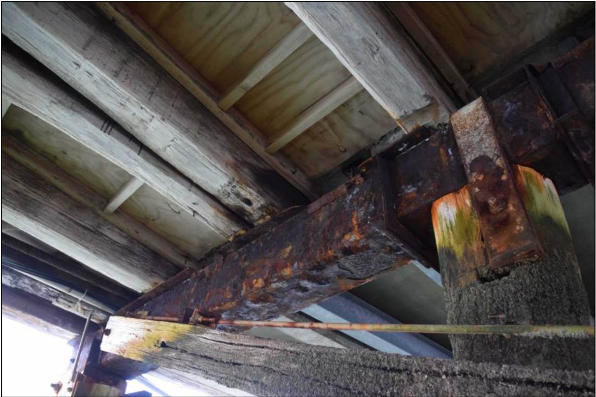
Photo 38 Severe corrosion to a past steel repair.
