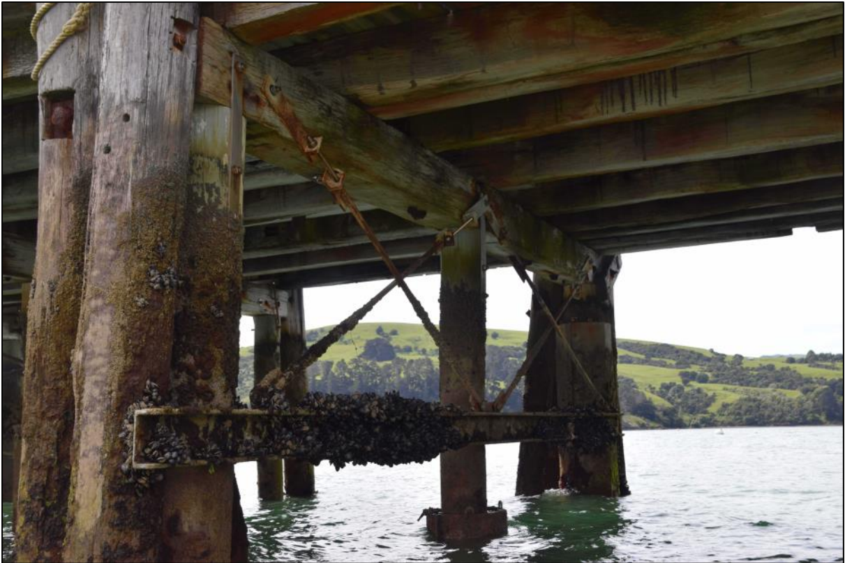
Photo 30 An example of modern steel repairs – bolted straps between the piles and cap beam, a steel PFC horizontal tie and double steel bracing rods. There is also an earlier steel jacket repair to the central pile.
