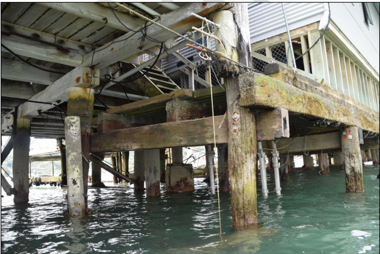
Photo 21 Between about bents 13 and 15 from the abutment, the south side of the wharf has been lowered in the past. None of the historic photographs show this lower and, hence, it seems to have been a 1970s or later alteration. In order to maintain the floor level, the corner of the modern shed (top right) has had to be built up on jack studs (with an area for services and plastic tanks below the floor). Note the steel props under the lowered deck.
