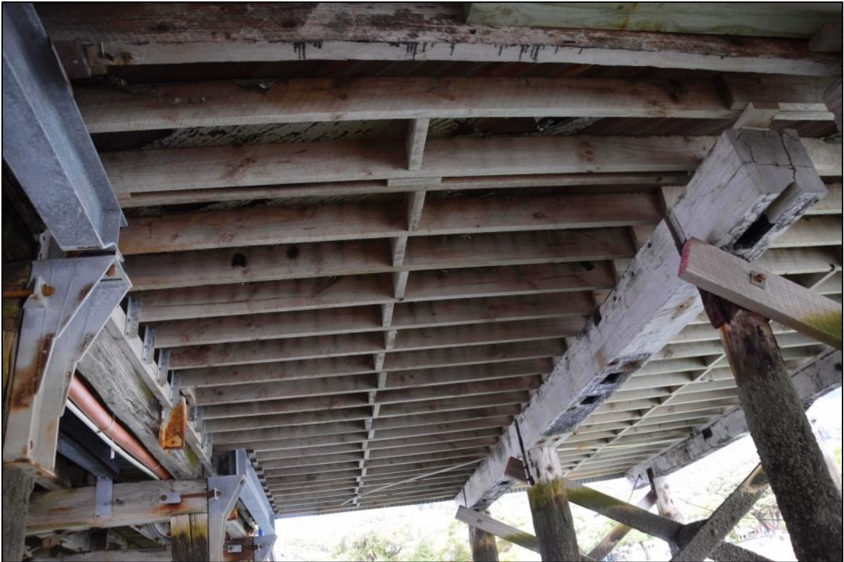
Photo 44 As Photo 43, but showing the more distant floor framing in greater detail.
