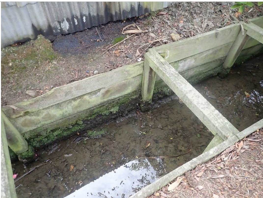
Figure. ii. Pollution of ground adjacent to the reach of Lydia Drain (7/9/18).
