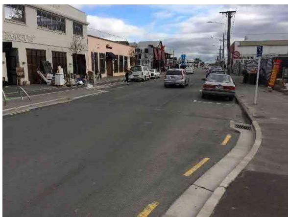
Photo 8: Centreline and RRPMs are worn and not visible, no edgeline guidance, vehicle driving in middle of road
