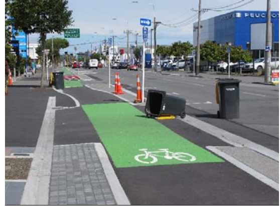
Photo 20: Rubbish bins placed in the parking shoulder. Note bins topple into cycle lane and block entrance.
