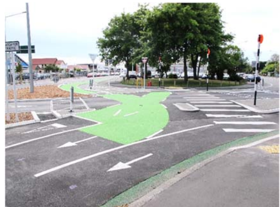
Figure 2-4: Actual controls and markings installed.
