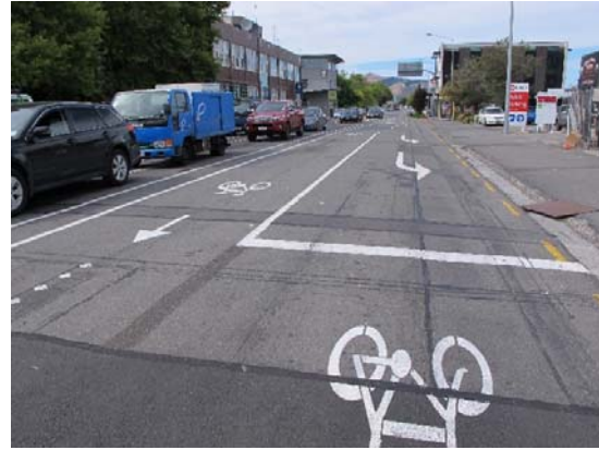
Photo 32: Lack of green markings – Madras Street.
