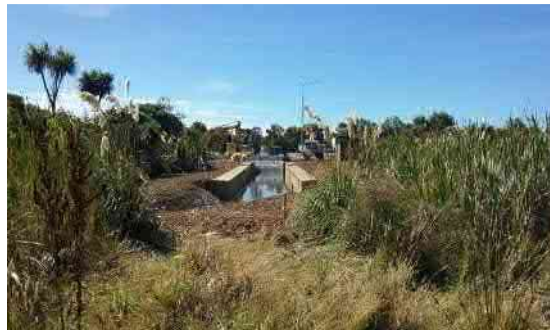
Image 2: Knights Pond & new Pump Station
