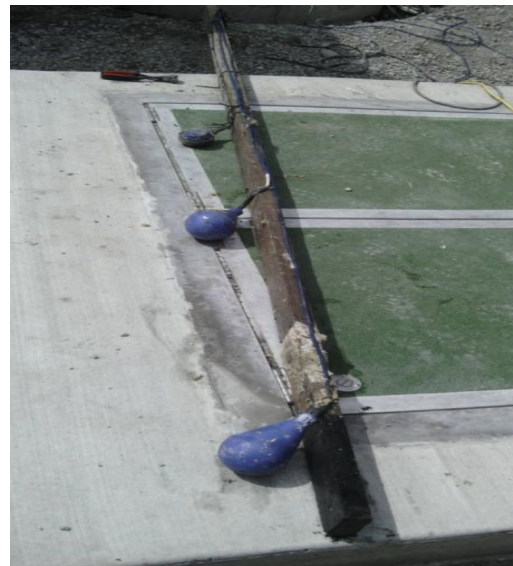
Figure 7: Electric Pump: Two Level Flow Switch
