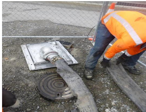
Figure 36: Manhole cover: Steel
