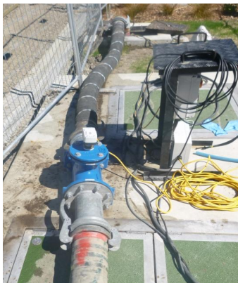
Figure 22: Flow Switch on Discharge Pipe
