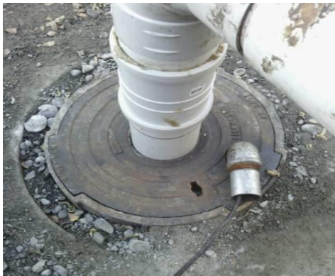
Figure 35: Manhole lid with PVC inlet
