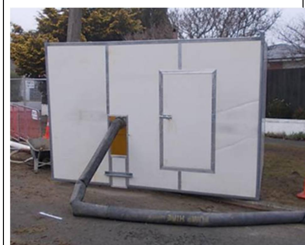
Figure 32: Noise Mitigation: Sound box
