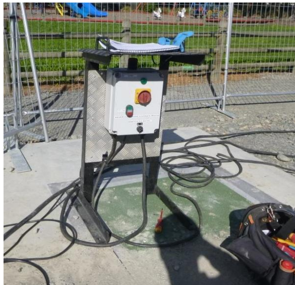
Figure 6: Electric Pump Builders Box
