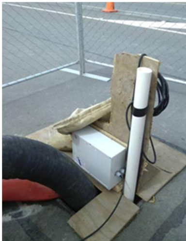
Figure 20: Float Alarm in Suction Manhole
