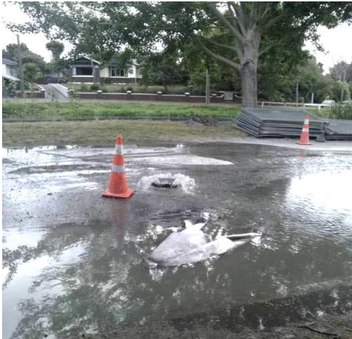
Picture 5. Wastewater overflow onto street due to pump station failure.
