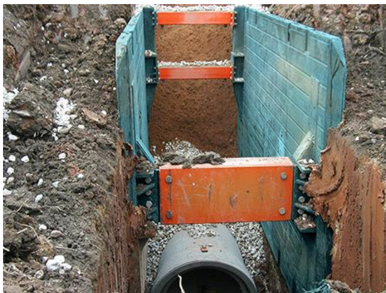
Figure 2-5 A Drag Shield can cut its way through native soil providing Positive Support
