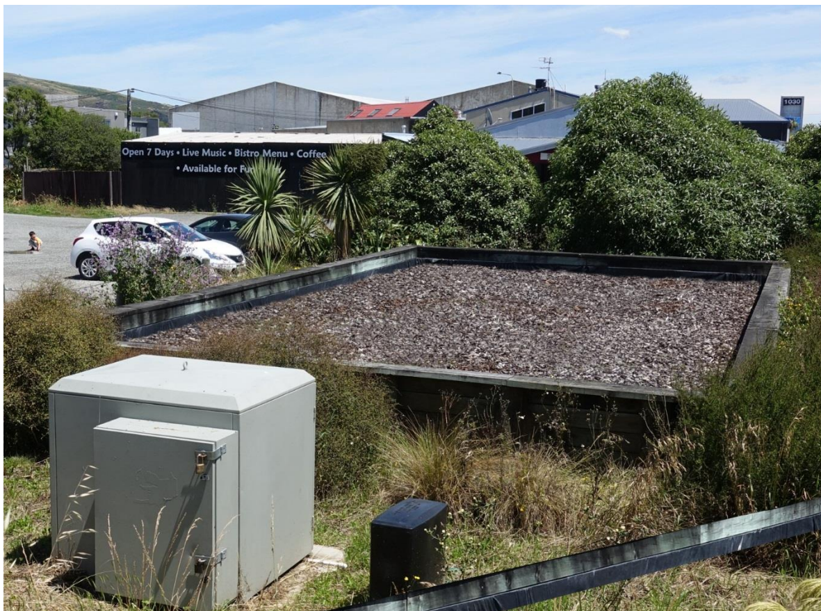
Photo: Ferrymead Biofilter for the PM57 discharge odours. Media almost entirely above ground level with a surrounding timber containment wall. Station ID OC0454.
