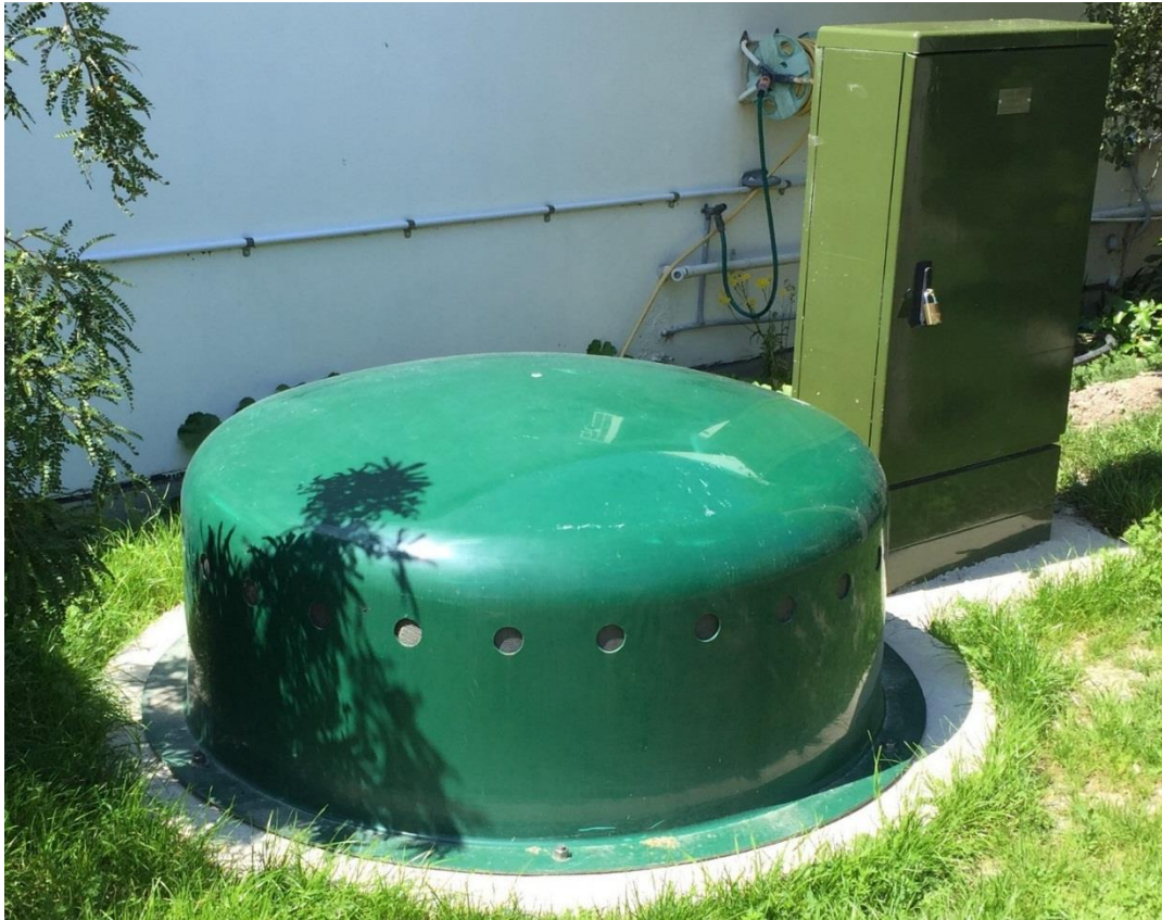
Photo: Settlers Crescent Carbon Filter for PM47 Discharge Odour Control – Station ID OC0501. Includes a 250mm wide concrete ring base pad to give an exposed concrete width of 150 mm.
