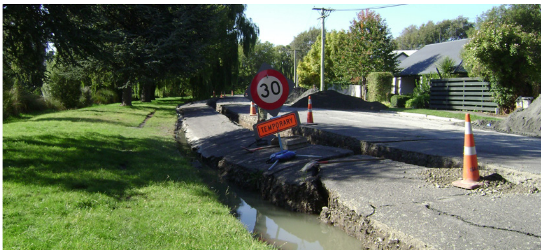
Lateral spread due to liquefaction
