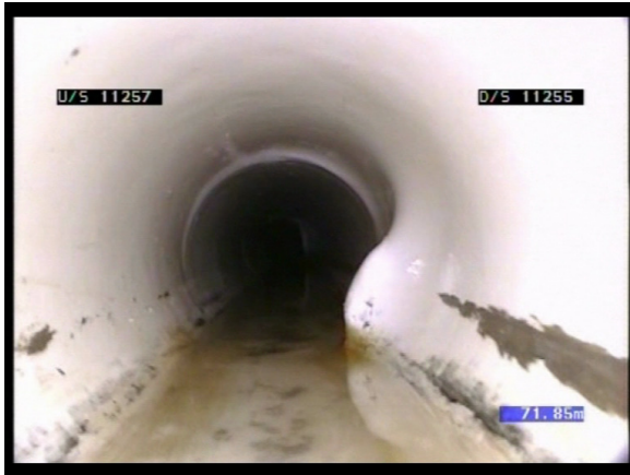
Large, bulge in the liner
