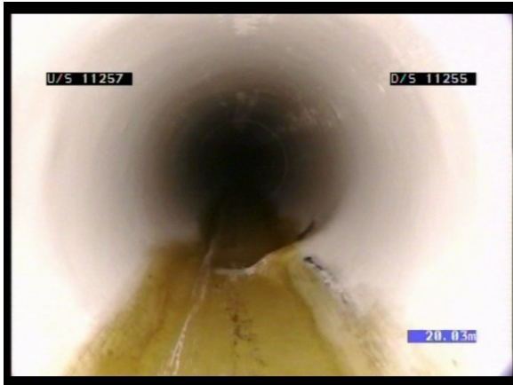
Medium, bulge in the liner.
