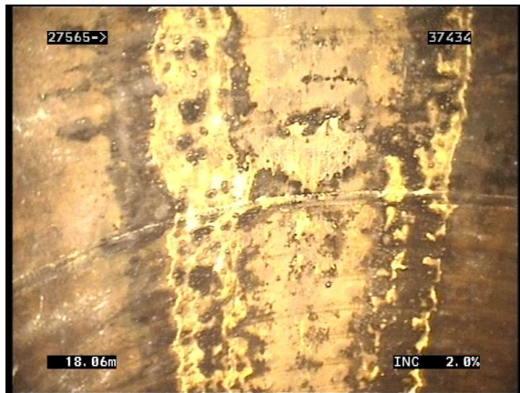
Photo, above, typical staining on the soffit (roof) of a liner, from the lubricants used during installation.
