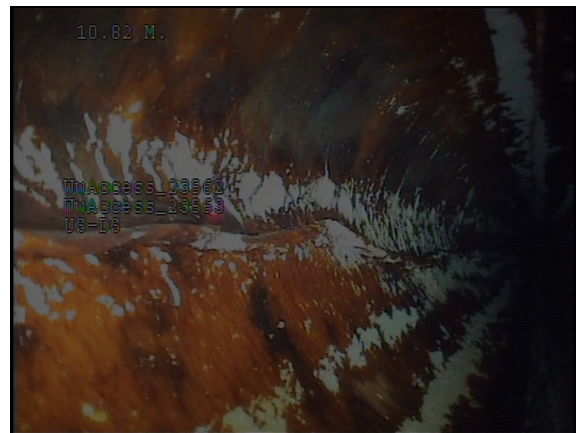
Small, longitudinal wrinkle on the side wall
