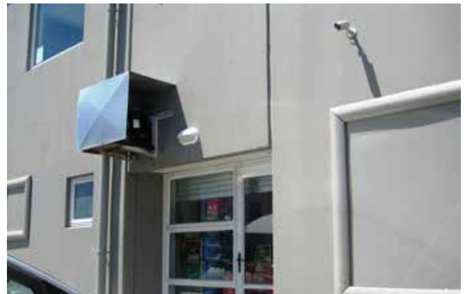
Example of CCTV at rear of premises
