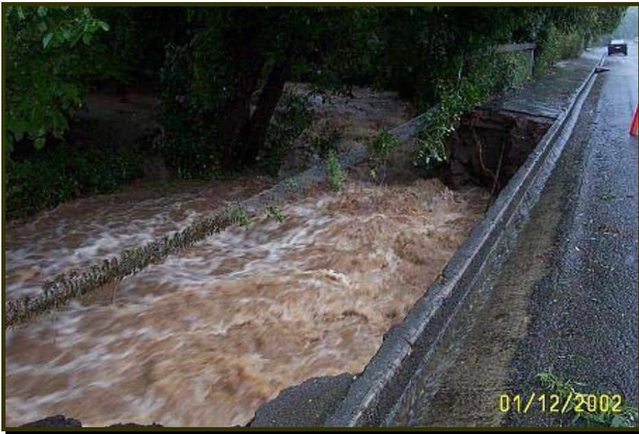
Balguerrie Stream along Rue Balguerrie opposite Muter Street showing footpath washed away. At the height of the flood water would have been flowing onto the street.
